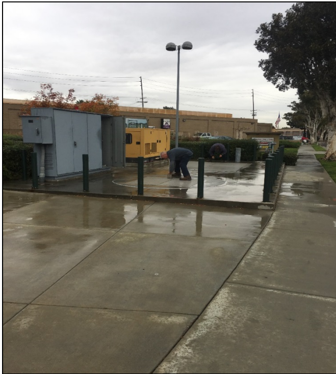
Photograph 7-5 Boeing Pump Station Pump Station Site
