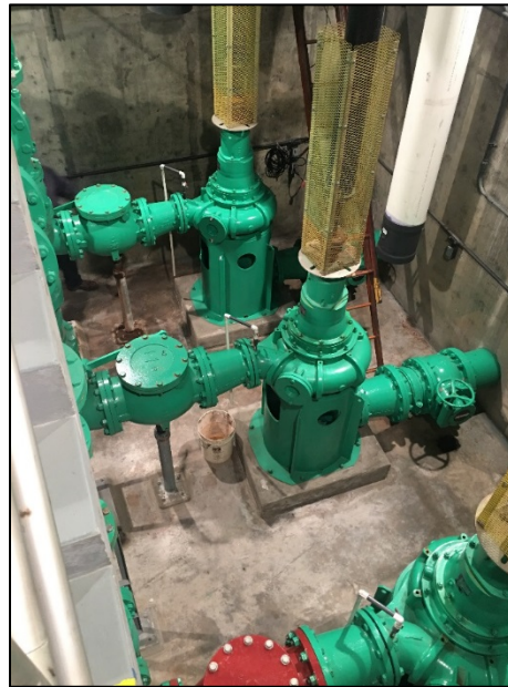
Photograph 7-15 Pump Station 35 Dry Well and Pumps
