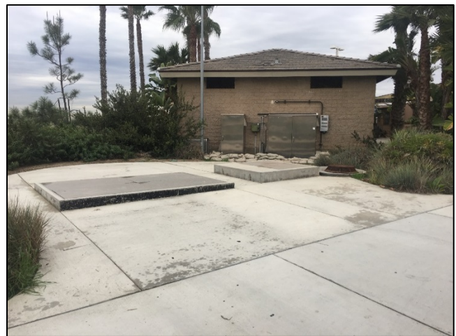
Photograph 7-13 1 st Street Pump Station Pump Station Site Concrete Paving after the 2007 Improvements
