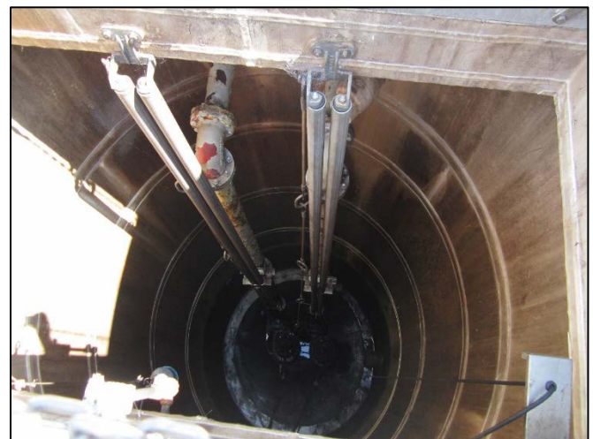
Photograph 7-2 Adolfo Lopez Pump Station Wet Well
