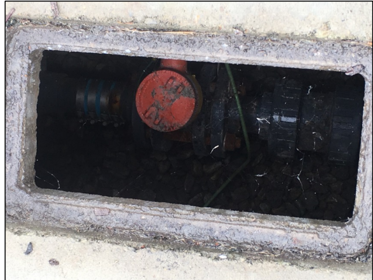
Photograph 7-4 Aquatic Park Valve and Meter Box
