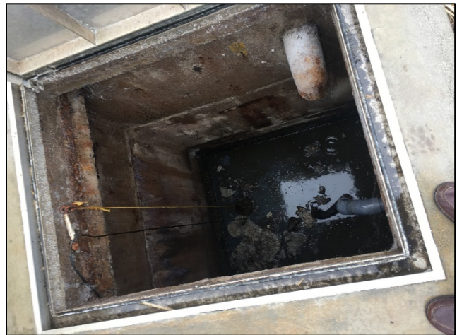
Photograph 7-3 Aquatic Park Pump Station Wet Well
